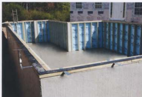
Salisbury-based Superior Walls of North Carolina supplied and installed the home's precast foundation.
